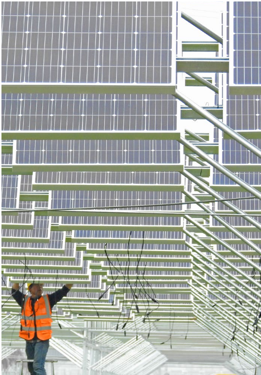
A worker installs solar panels at a photovoltaic power station in Lianyungang City (Jiangsu province, 2018).
