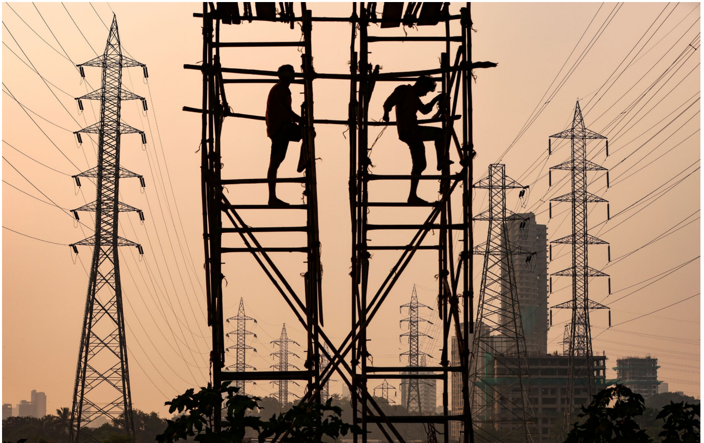
Labourers work on scaffolding set among high tension electricity pylons in Mumbai (October 2021).
