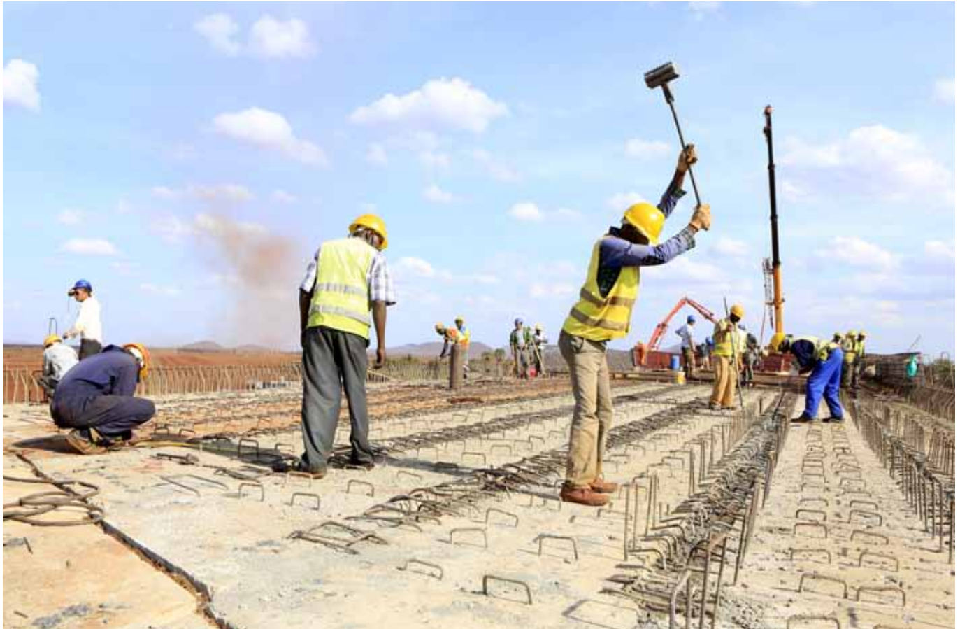
Workers laying track at an overpass bridge at Emali, Kenya, on the Mombasa-Nairobi standard gauge railway. Africa is a focus of BRI activities.
